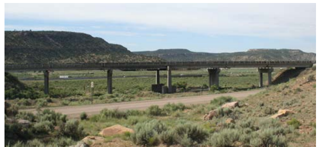
Constructed in 1950 and listed on the National Register of Historic Places and the New Mexico State Register of Cultural Properties as part of Route 66, BHI replaced the steel girders and straddle bent with new steel framing and a joint-free deck.
